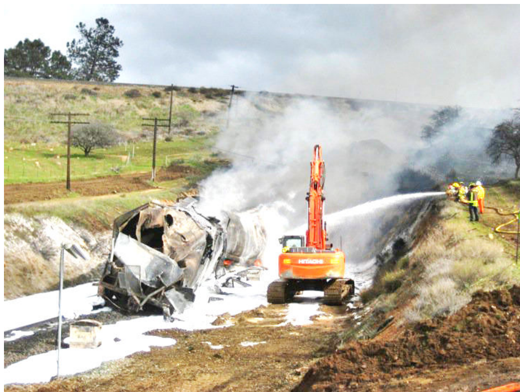
The south portal of Tehachapi tunnel on Feb. 22, the morning of the second day after the initial call. The cars have been removed from the tunnel and the fire is under control. Soon the railroad will begin clean-up and replace the track inside the tunnel
