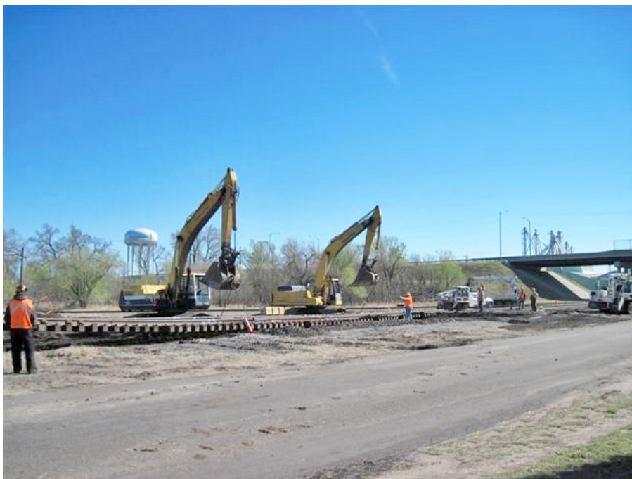
Tuesday, April 5, UP was installing a new turnout for the west "City" switch in Hutchinson. This is part of a project replacing 33 miles of 112 lb. jointed rail with 136 lb. welded rail between Arlington and Groveland. Photo by Lynn Aldrich.
