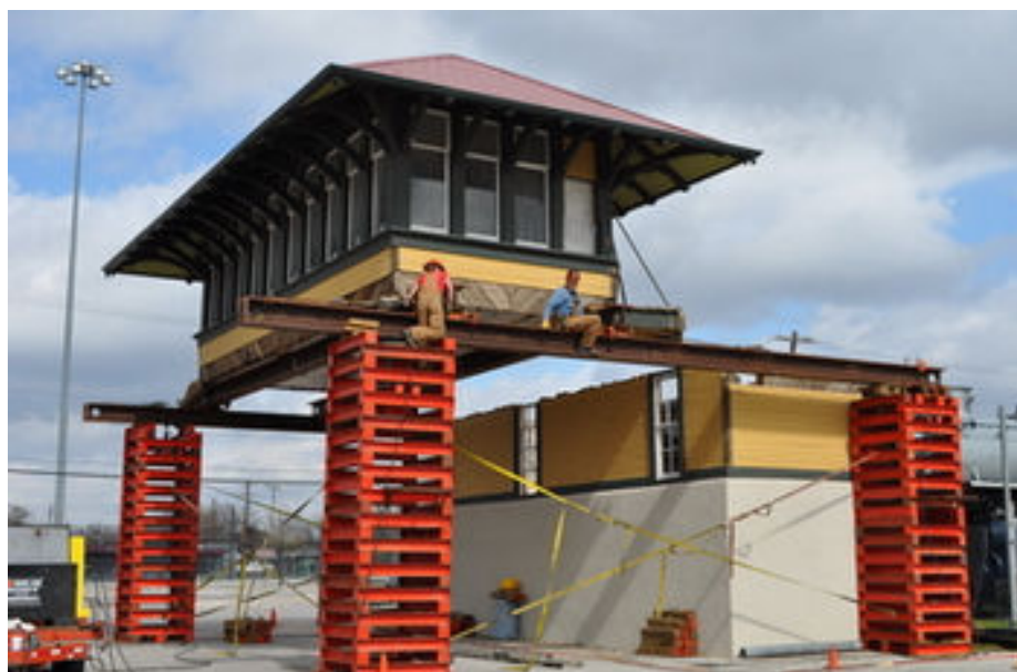
Movement of Tower 19 required dismantling the three story structure. The tower was moved to Fair Park in 1996.
